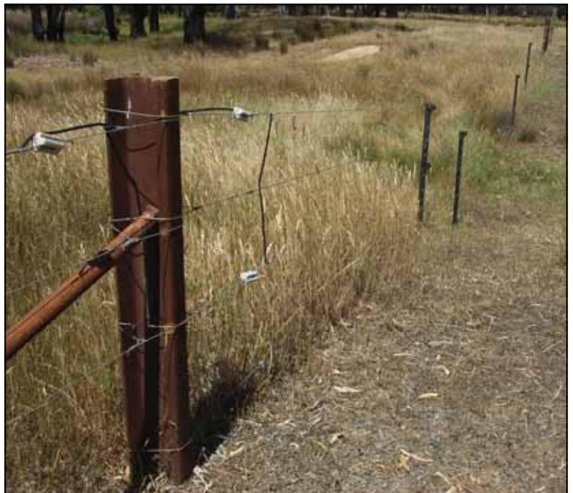
Photo 2: End assemblies are the most expensive part of a fence to install. A flood channel crosses this fence from left to right, & this length has been wired as a separate "sacrificial" section (note the end assemblies each side of the channel). Each section of the fence between the posts have been wired separately (note the wiring at the post in the foreground).
